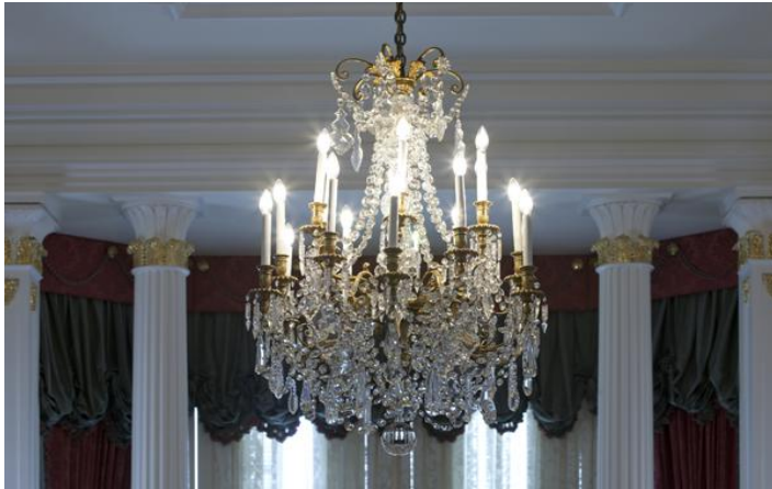
Borealis B10 LED Candelabra Lighting Installation
